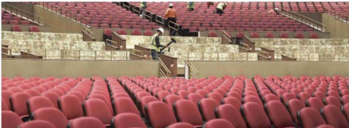
Workers prep the new live performance theater. The plan to overhaul the Hollywood property called for the demolition of the old live-music venue and its outdated, outdoor festival-style mall. The casino floor was expanded and refurbished.
