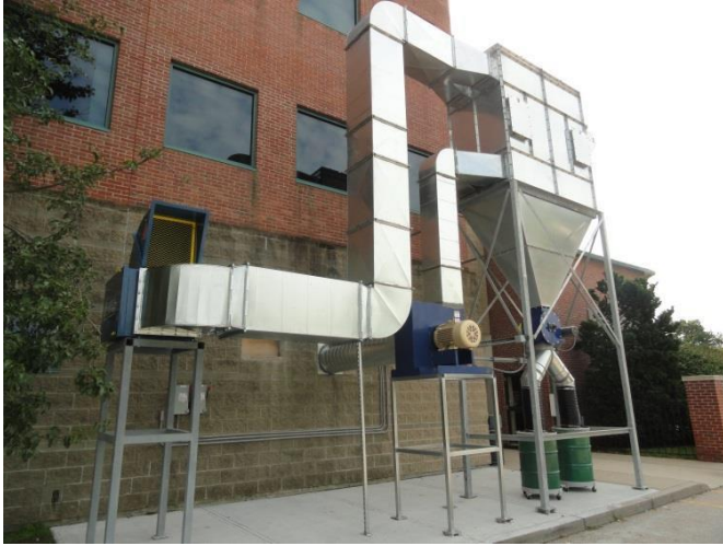
30 HP Drum Storage
