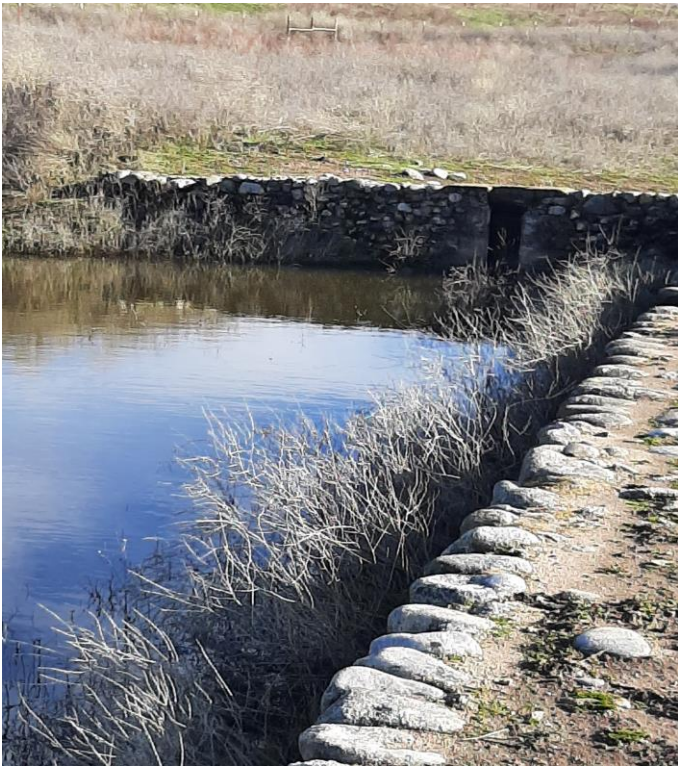
The Mill Pond Reservoir full of water! The stone wall is part of the original mission water system developed in the 1770s.
