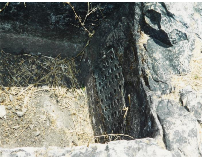
Photograph of the metal grate at the Noria Reservoir
